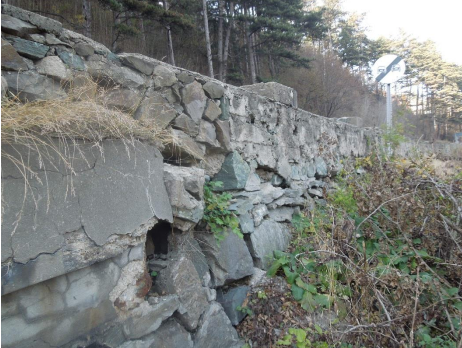
Fig. 1 Elemente constructive aflate in stare avansata de degradare
