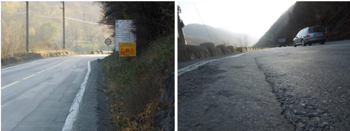
Fig. 2 - 3 Elemente constructive aflate in stare avansata de degradare
