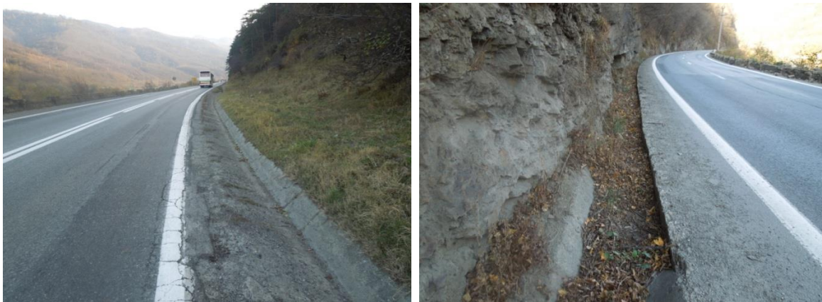
Fig. 6 - 7 Elemente constructive aflate in stare avansata de degradare
