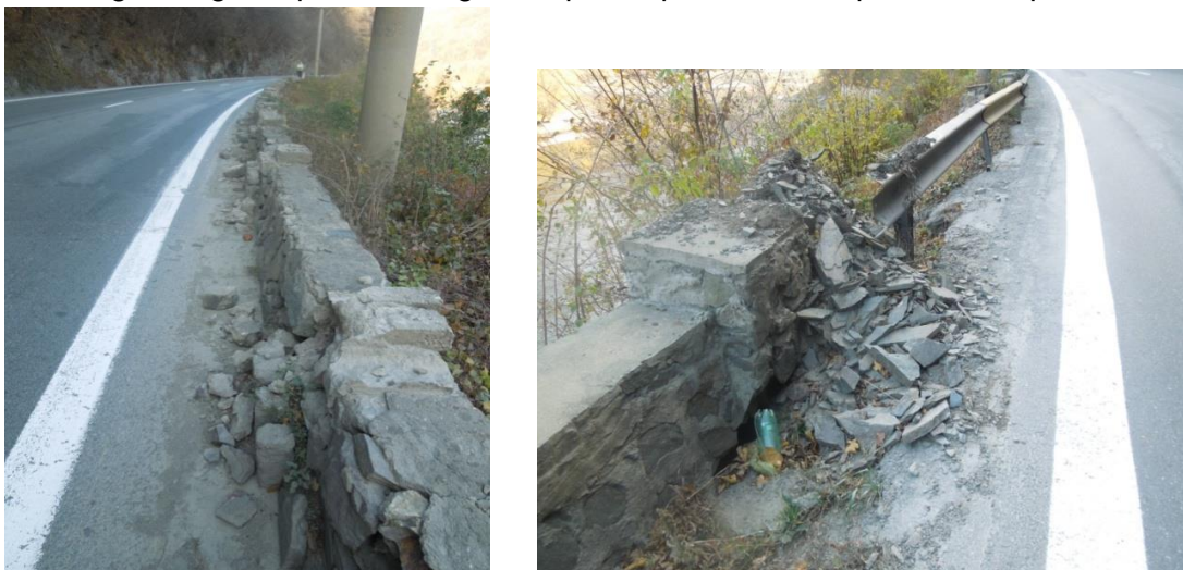
Fig. 13 - 14 Elemente constructive aflate in stare avansata de degradare
