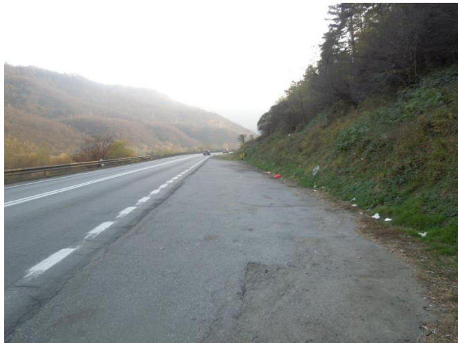
Fig. 8 Elemente constructive aflate in stare avansata de degradare
