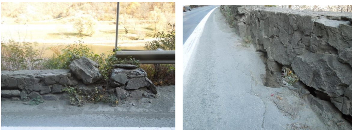
Fig. 11 - 12 Elemente constructive aflate in stare avansata de degradare
