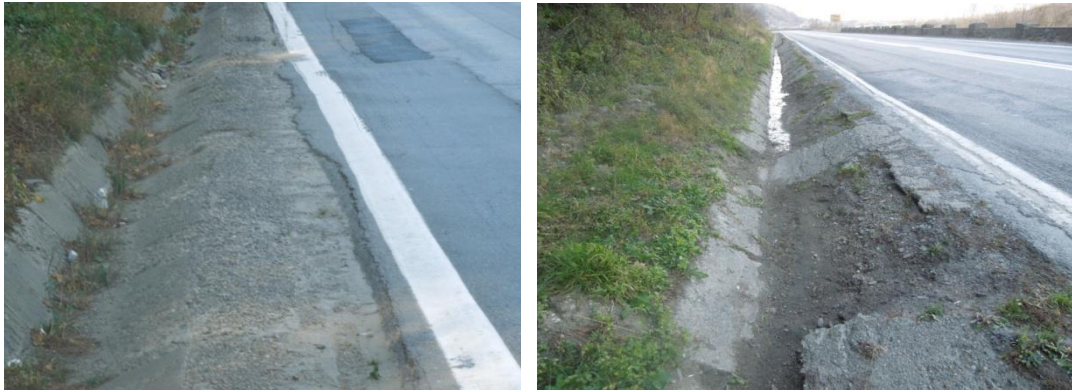
Fig. 4 - 5 Elemente constructive aflate in stare avansata de degradare
