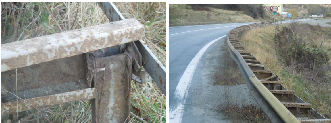
Fig. 15 - 16 Elemente constructive aflate in stare avansata de degradare
